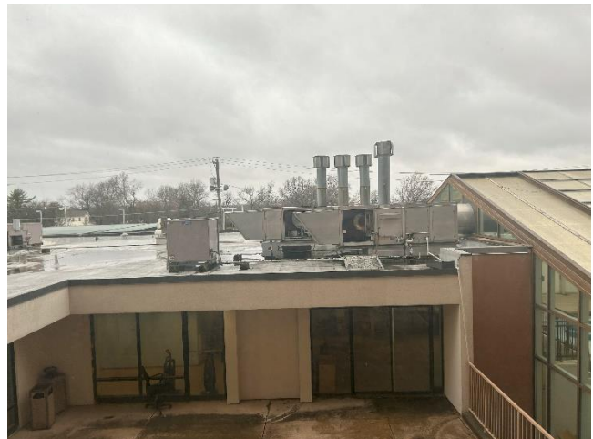
Right: An image of the inoperable air handles associated with the pool building.
