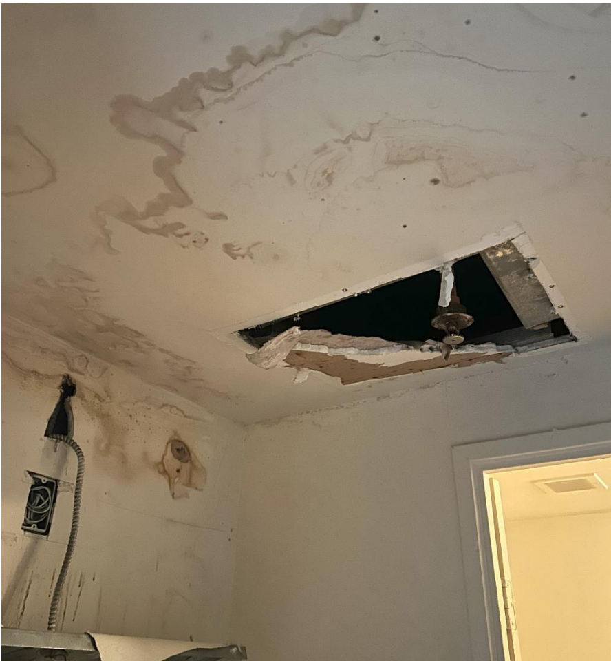
Above: Water damage and mold in the interior of the Hotel.
