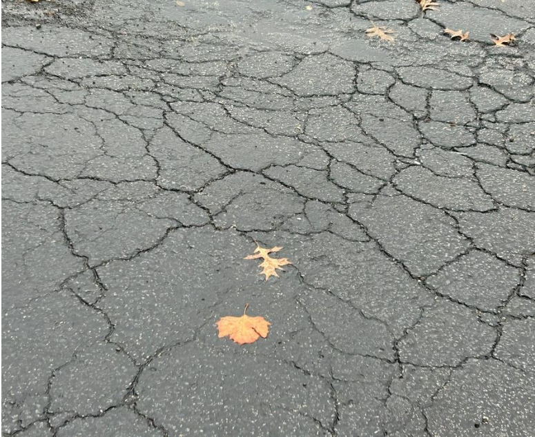
Above and below: Deteriorated asphalt pavement.
