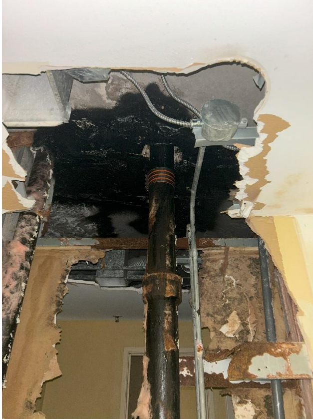
Left: Evidence of interior hotel room water damage.
