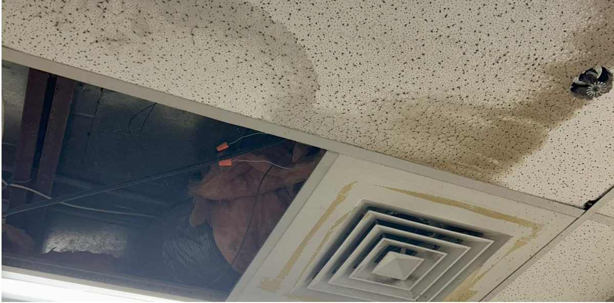
Above: Water damage in the interior of the Hotel.
