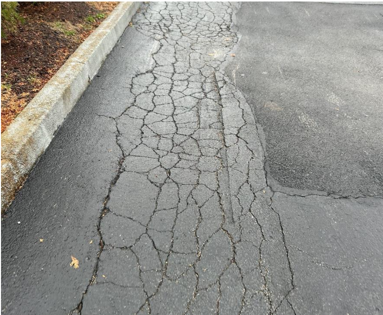
Above: Deteriorated runway.
