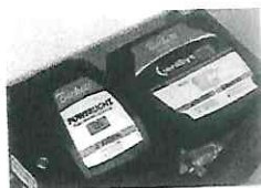
Diesel fired Beckett Burner
